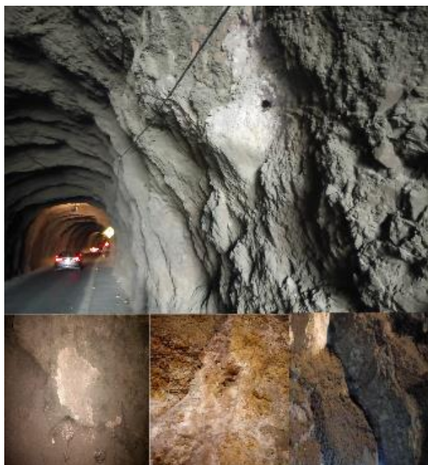
Fig. 5. Details of sampled wall tunnels. The biggest panel shows a general view of one tunnel while the smaller point specific sites where the wall samples were scraped.
